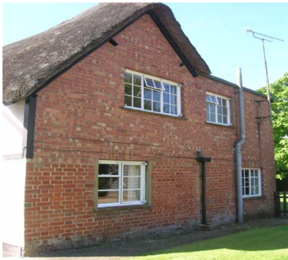
Below: An unsympathetic flat roofed extension with unsightly waste pipes, modern windows and aerial
